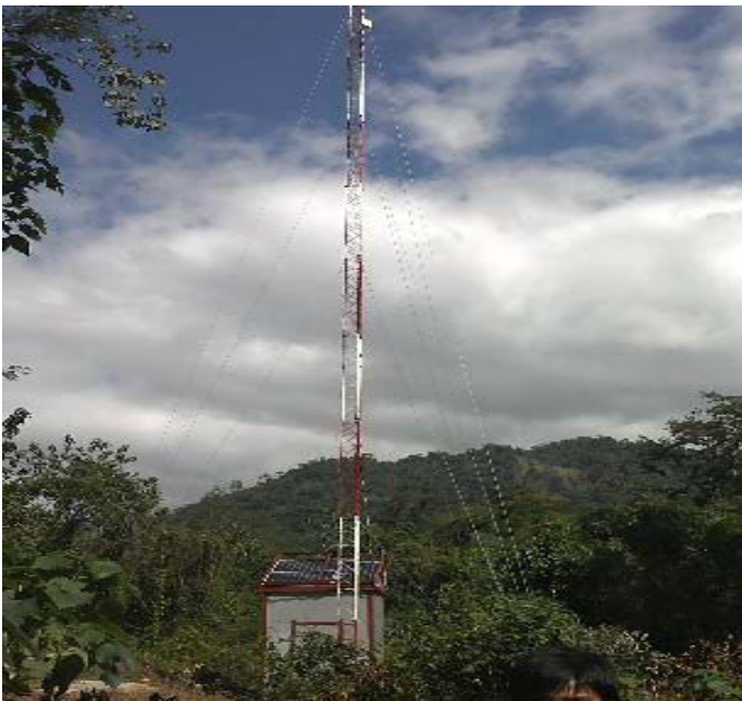
Rain gauge on the basin, with surveillance camera and sound-alert system to protect the system at Da Ban reservoir, Southern Vietnam
