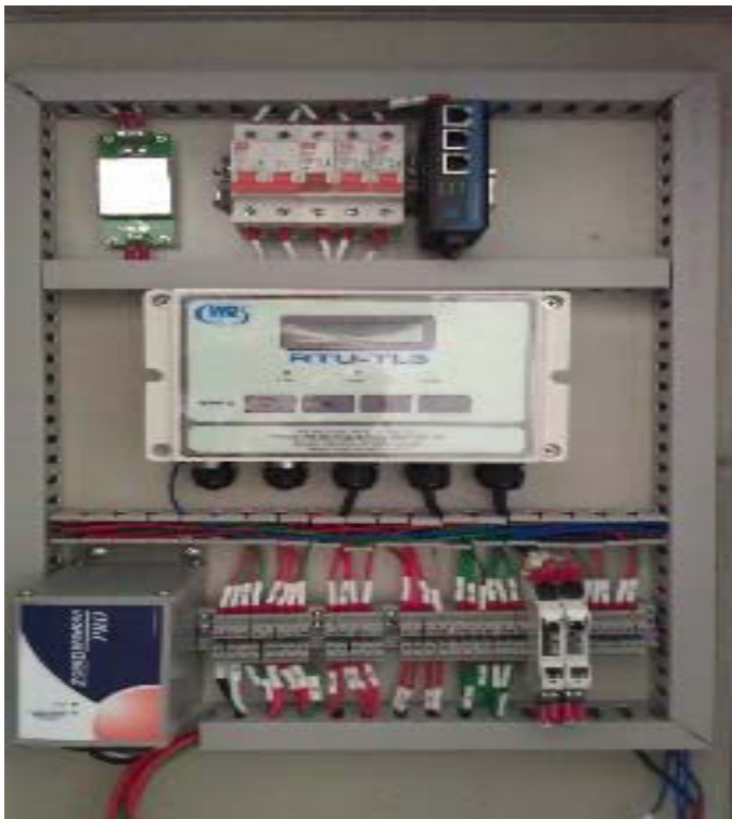
Inside of a monitoring cabinet at IaMla reservoir's spillway, Highlands of Vietnam
