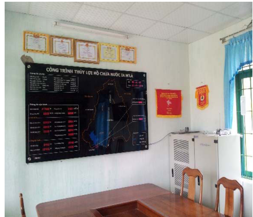
Electronic board and central monitoring cabinet in IaMla reservoir, Highlands of Vietnam
