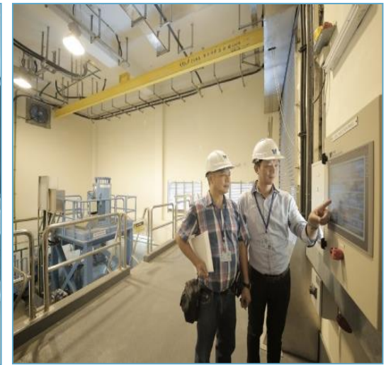
Operation of Hydropower Plant via its Local Control Panel
