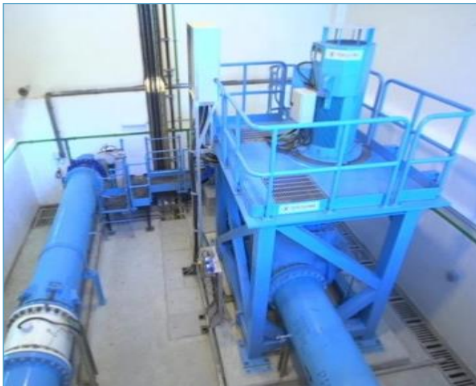
1 st set of Hydropower Generator up and running in 2013
