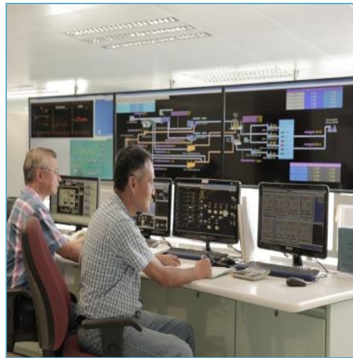
Operator at Central Control Room of Water Treatment Works
